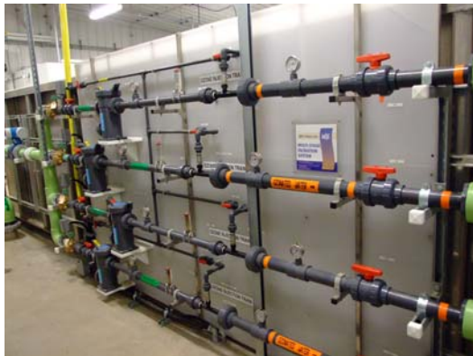
Ozonation Injection System
