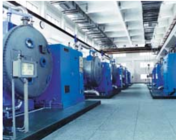
Water work Deoksan, Pusan City, South Korea Capacity: 203 kg ozone per hour
