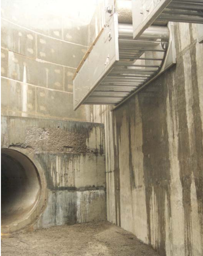
Inchcape (Pump Station), UK, 69 mgd (3,000 l/s)
