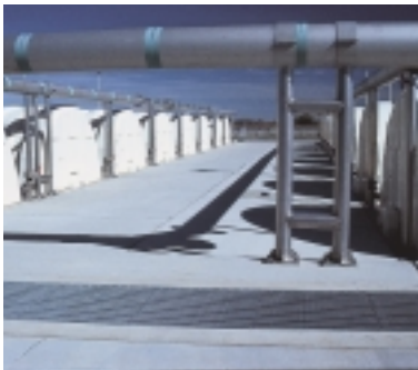
This RBC plant can be provided with supplemental air to reduce maintenance and energy requirements.
