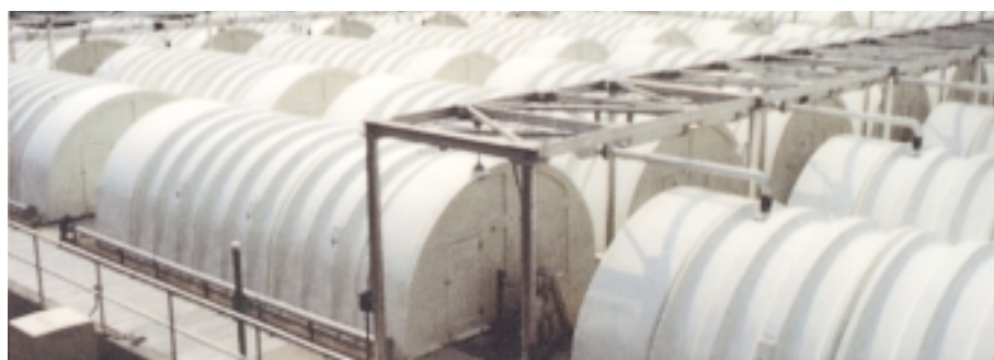
Series 300 RBCs have served this 27 MGD plant for more than 10 years.
